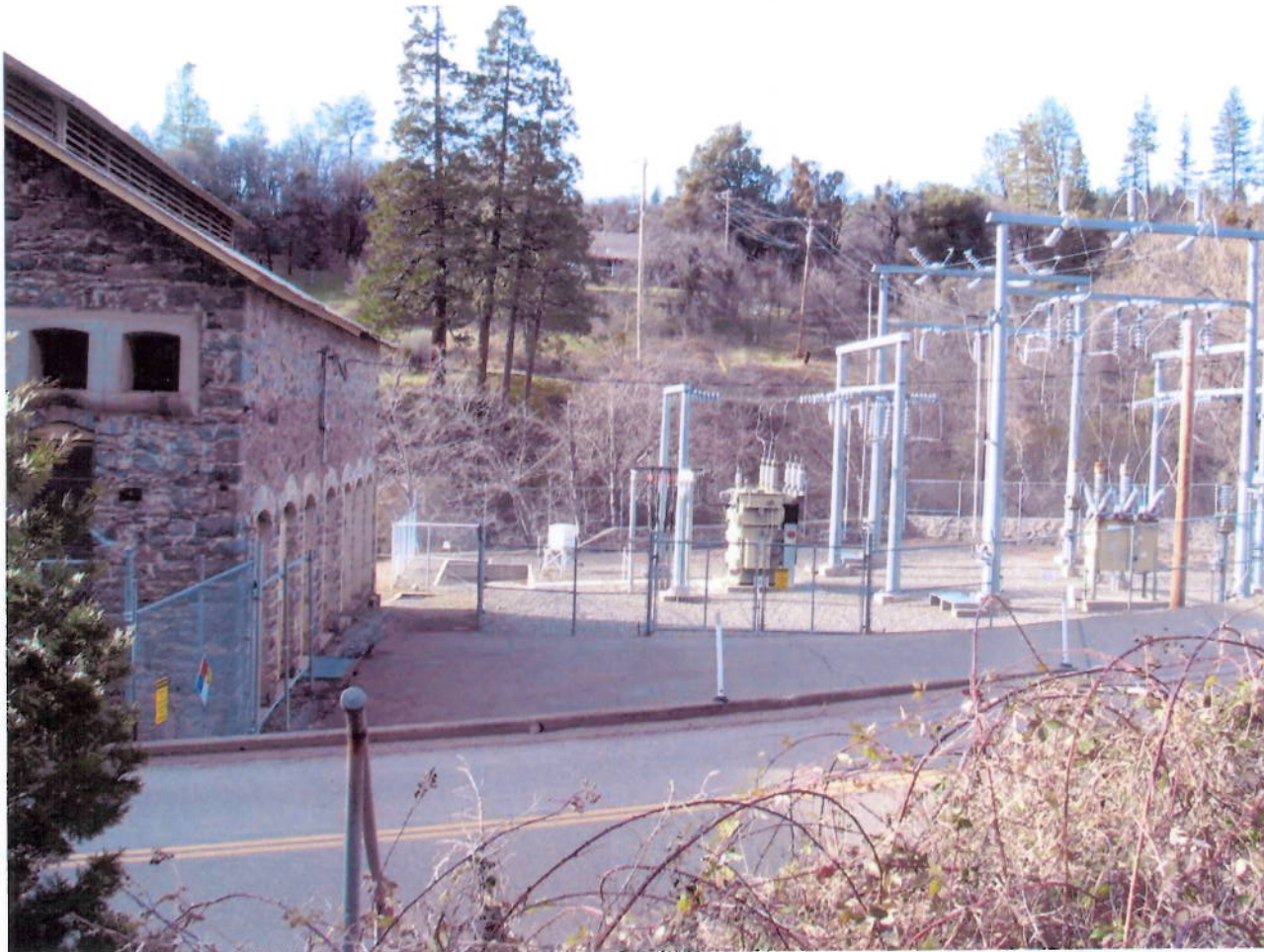
Kilarc Powerhouse and Switchyard
